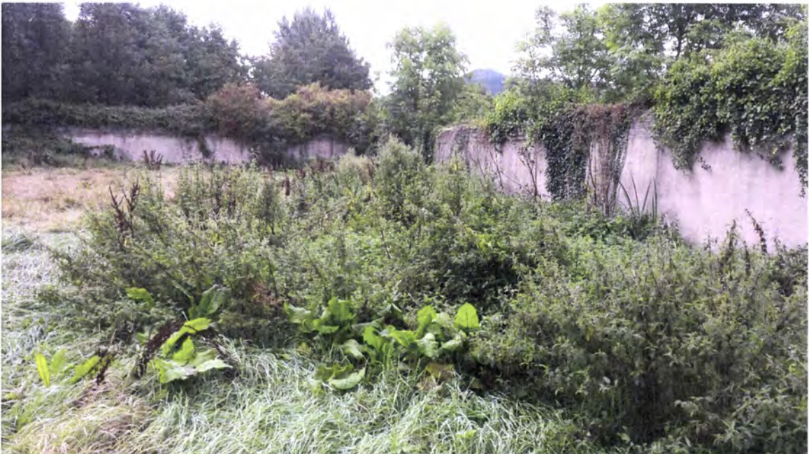
View of the west side of the site with the stream bank behind the block wall
